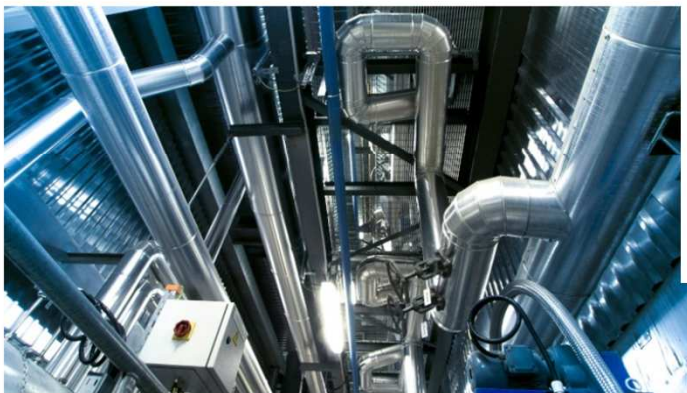
ExxonMobil's facility in Gravenchon processes 425,000 t/y of ethylene
